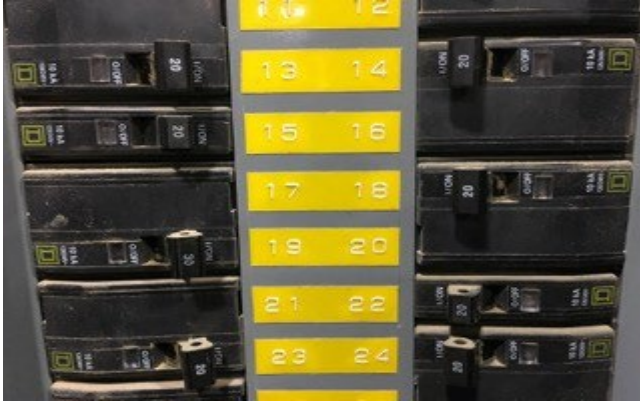
Image No. 3 – Enlarged view of Panel S2, Breakers 13-24
