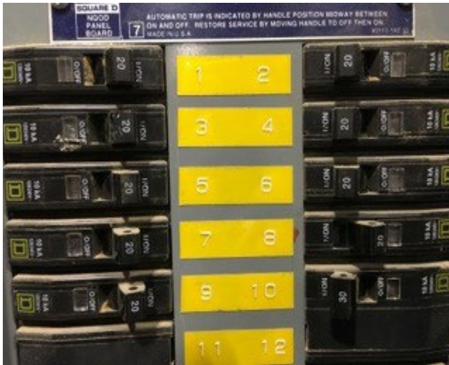
Image No. 2 – Enlarged view of Panel S2, Breakers 1-12
