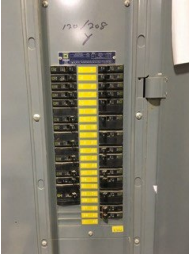
Image No. 1 – Existing Panel S2 Overall
