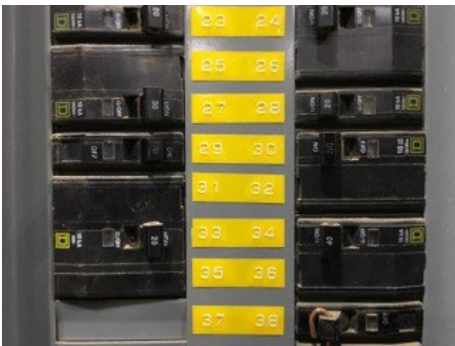
Image No. 4 – Enlarged view of Panel S2, Breakers 23-38
