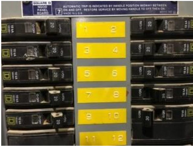
Image No. 2 – Enlarged view of Panel S2, Breakers 1-12
