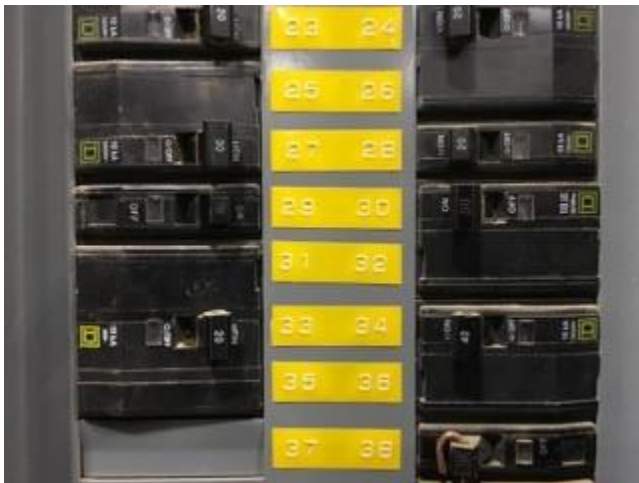
Image No. 4 – Enlarged view of Panel S2, Breakers 23-38
