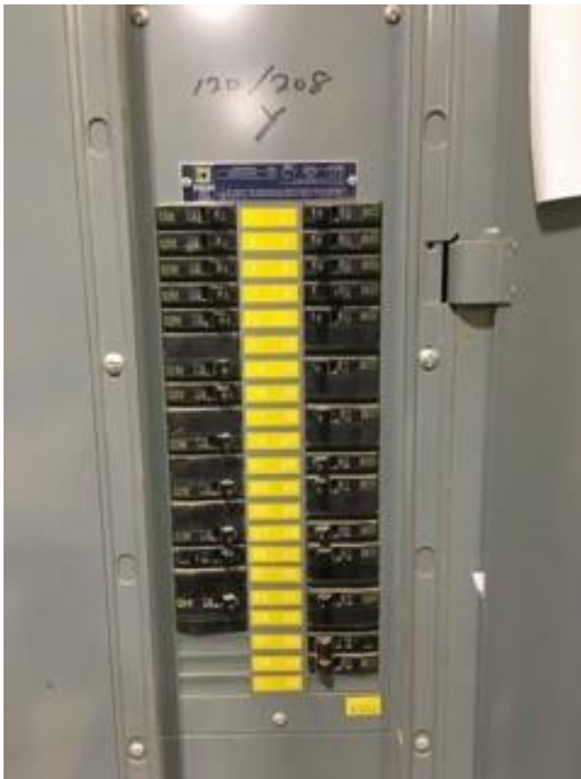
Image No. 1 – Existing Panel S2 Overall
