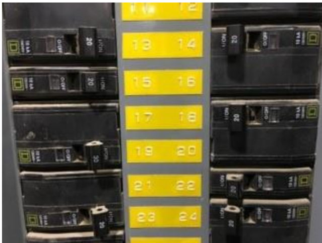
Image No. 3 – Enlarged view of Panel S2, Breakers 13-24
