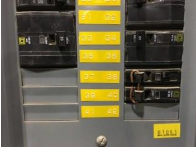
Image No. 5 – Enlarged view of Panel S2, Breakers 31-42
